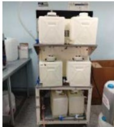
Figure 39 Solvent recovery / recycling systems CBG
