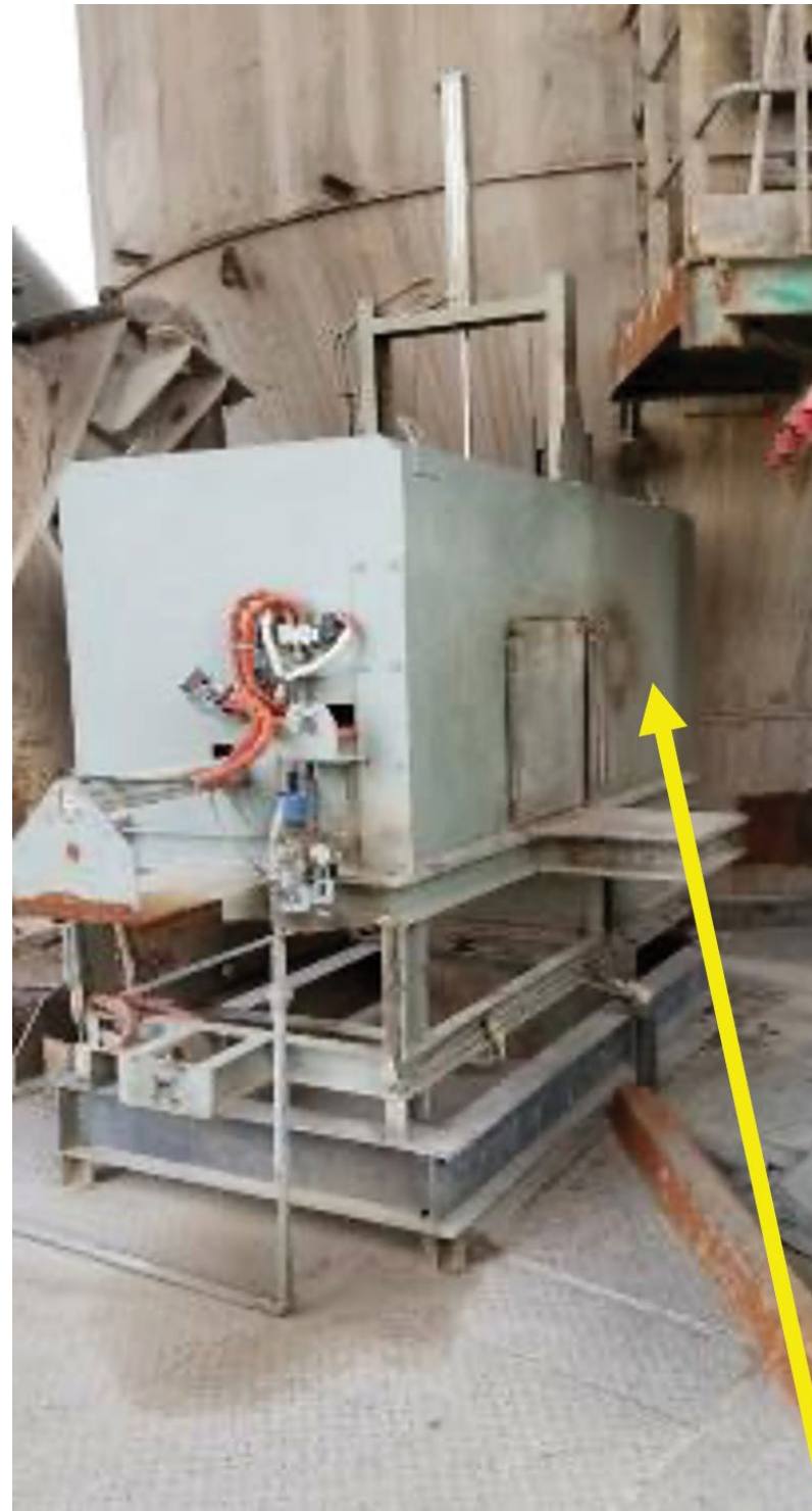
Ram feed for waste containers
