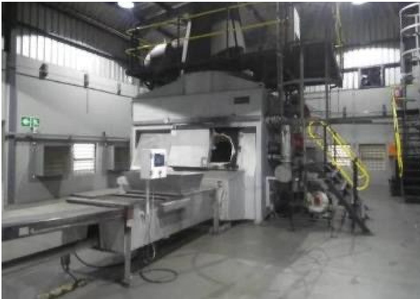
Modern High-temperature incinerator with ram feed
