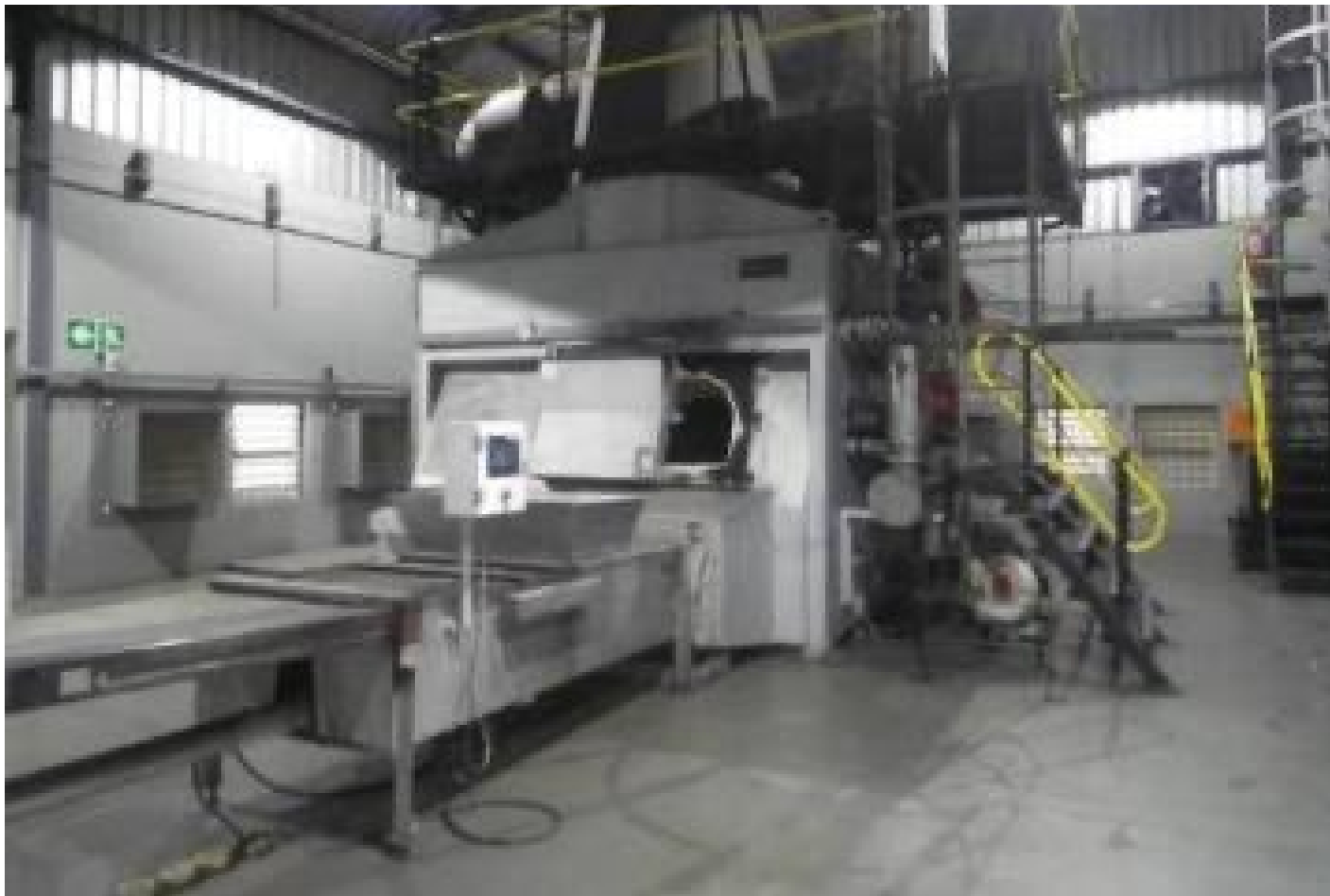
Modern High-temperature incinerator with ram feed
