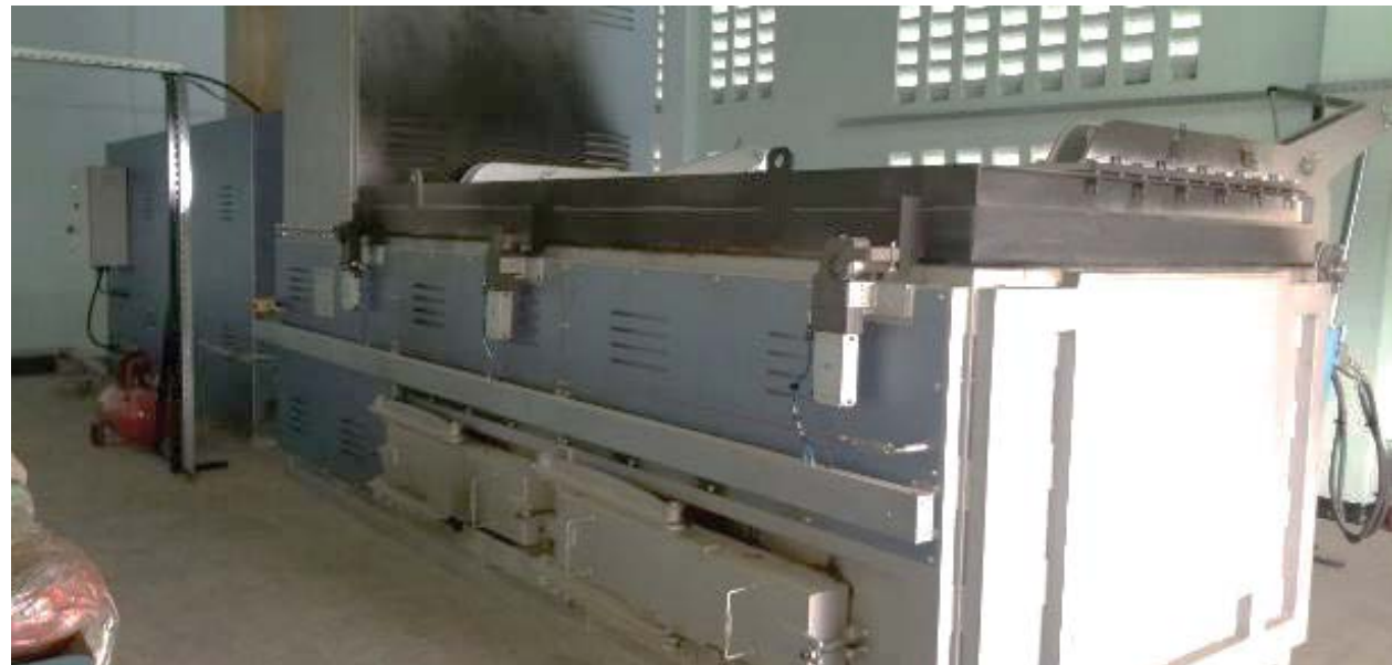
Figure 23 Fixed hearth incinerator - Inciner8
