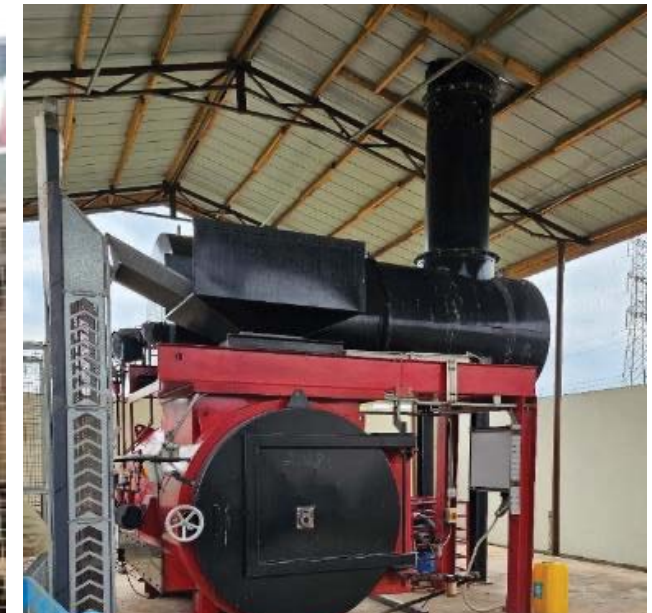
Figure 25 Fixed hearth incinerator - Addfield
