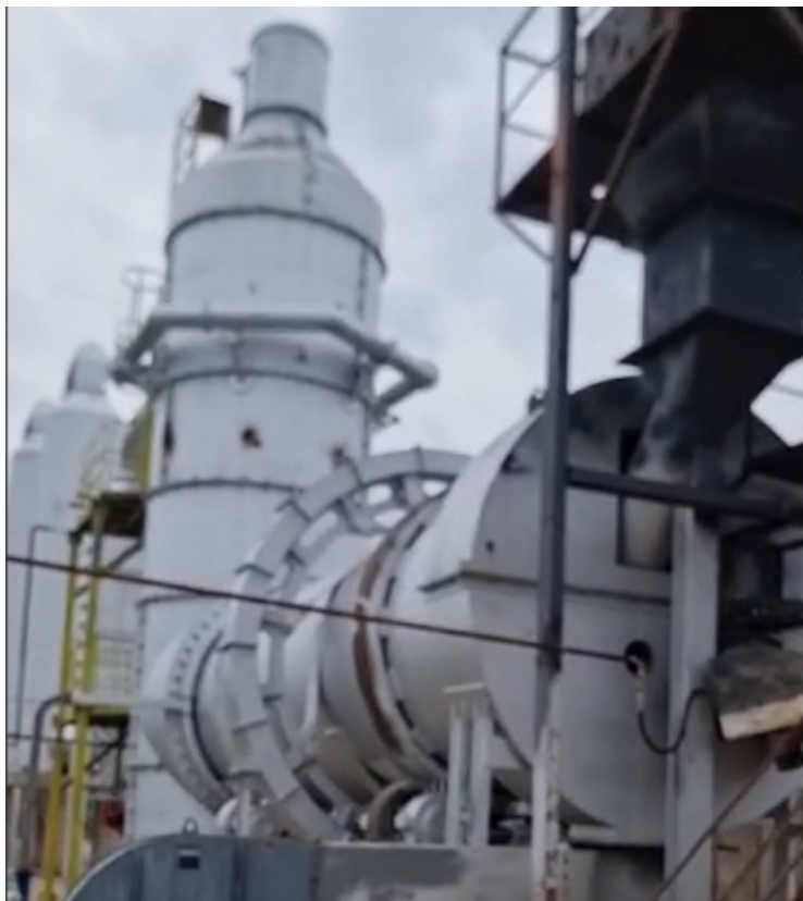
Figure 26 Rotary kiln incinerator
