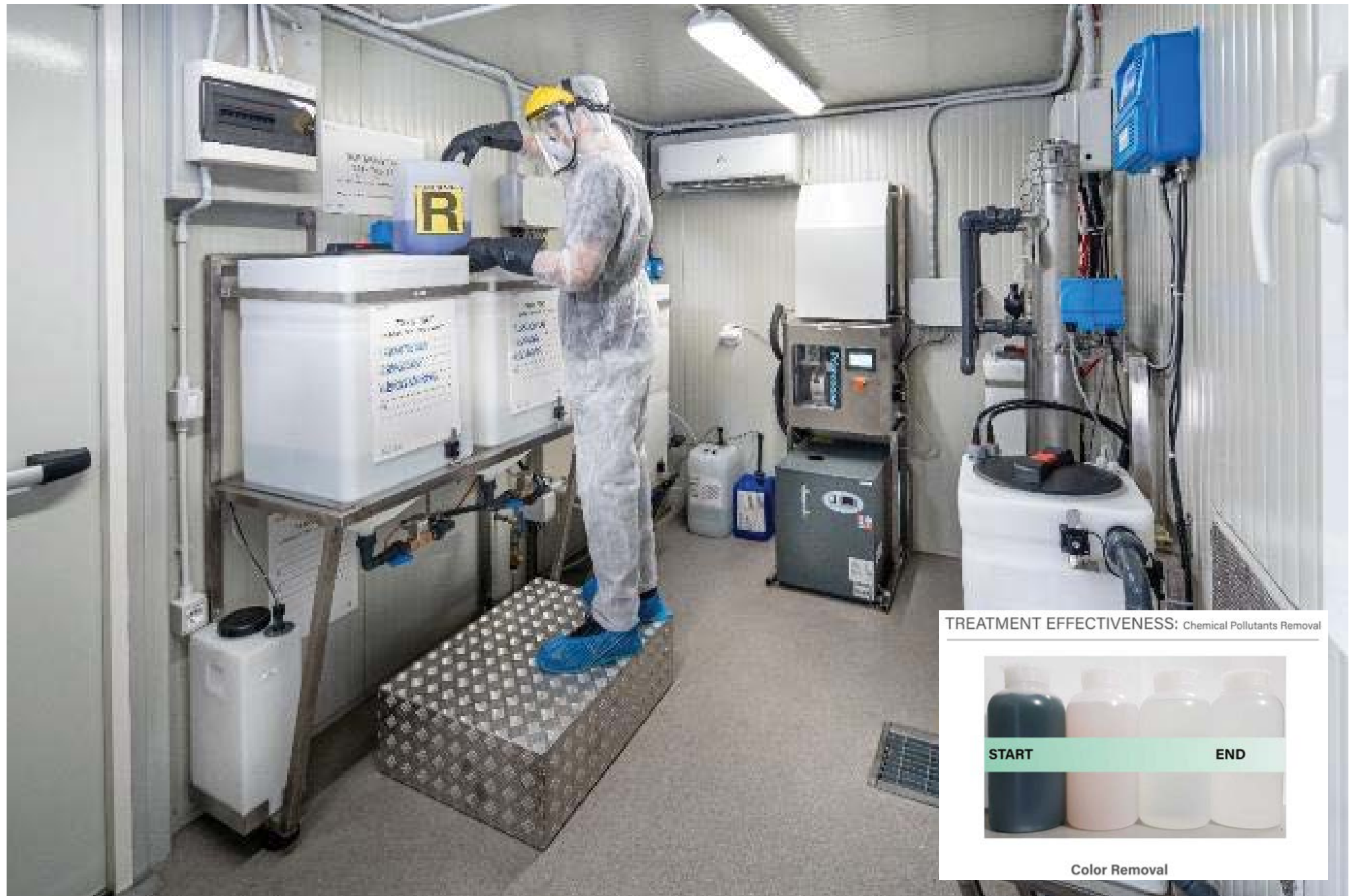
Figure 37 Newster PURA chemical waste treatment system
