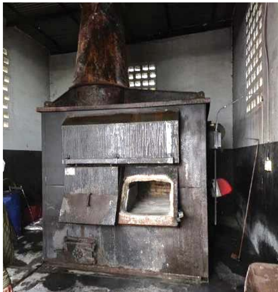
Figure 22 Fixed hearth incinerator - SA Incinerator
