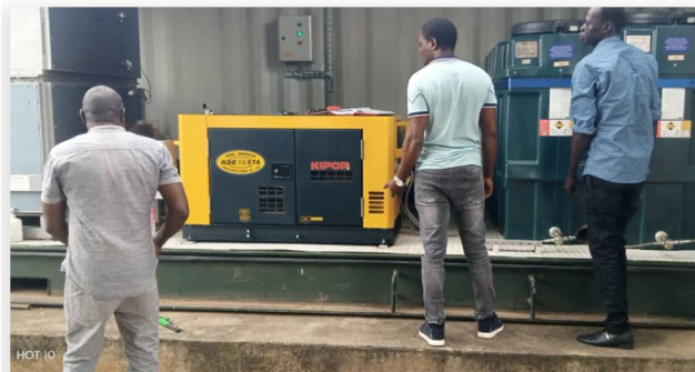
A full inspection of the installed and commissioned high capacity incinerator
